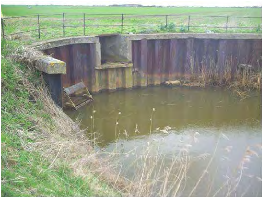
Plate 72 The sluice on Bosky Dyke (Keadby Warping Drain) near Keadby (source: HIFI)
