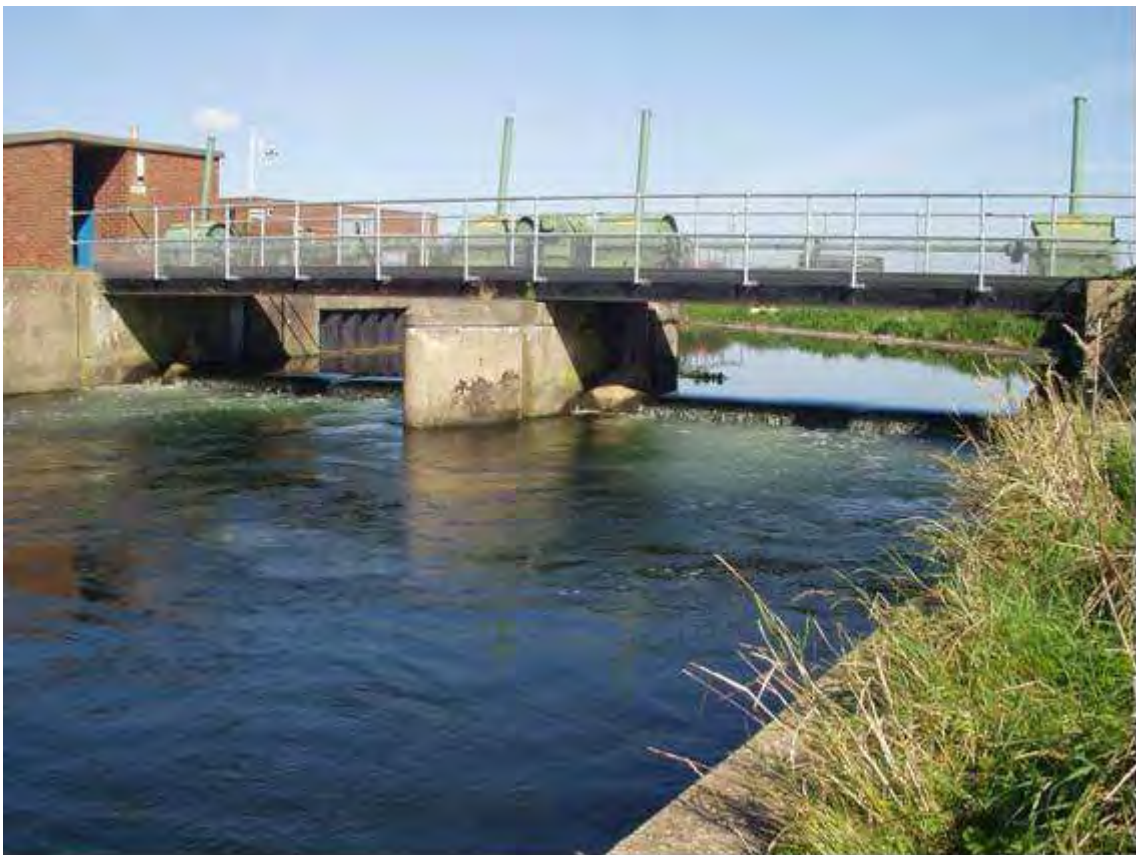
Plate 2 Hempholme Weir (at high tide) on the River Hull (source: Environment Agency)
