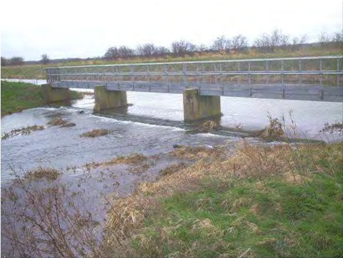
Plate 58 Harlam Hill Weir (u/s) on the River Ancholme (source: HIFI)
